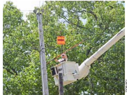
Crew members from Arkansas and 10 other states restore power after Memorial Day weekend tornadoes in northern Arkansas.
